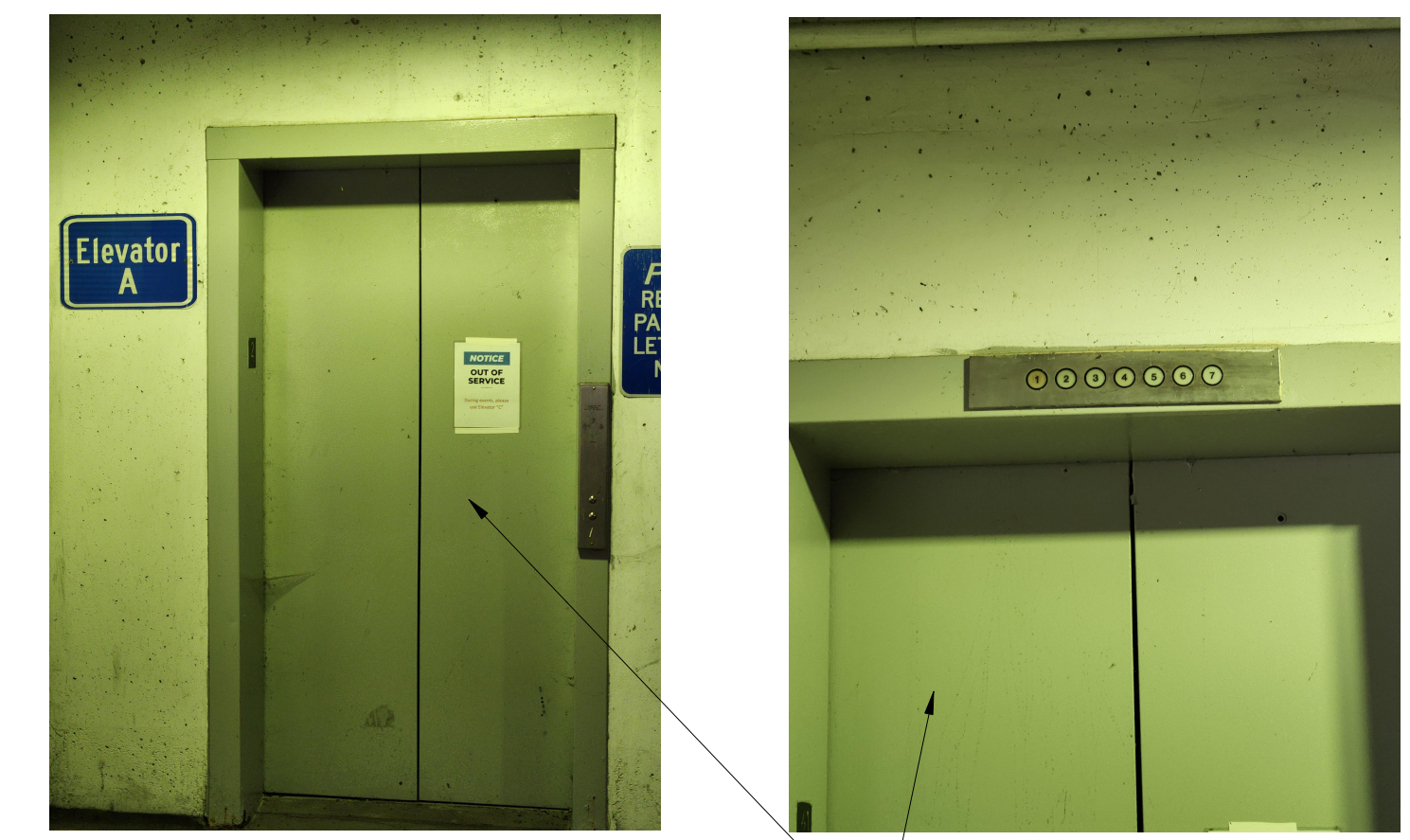
TYPICAL EXISTING HOISTWAY DOORS THE PHOTOS ARE TYPICAL FOR THE VARIOUS FLOORS AND ARE PROVIDED FOR INFORMATION
