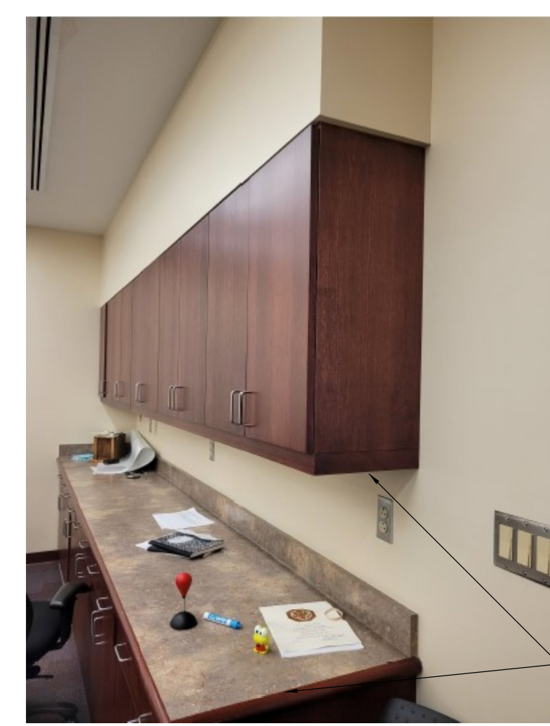
(E) BASE CABINETS, COUNTER TOP, AND WALL MOUNTED CABINETS TO BE REMOVED
