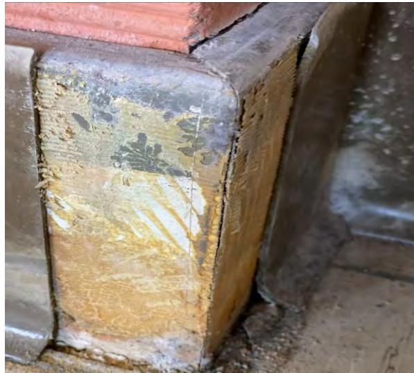
HA 11 - Tan Mastic from Tan Non-Suspect Vinyl Cove Base, No Asbestos Detected
