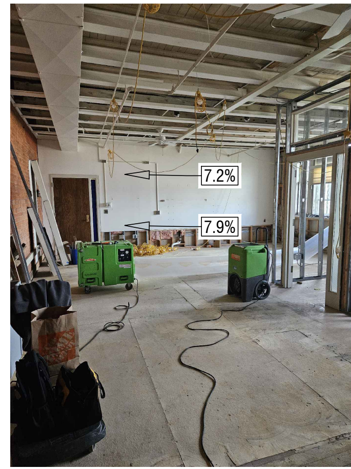
B SLM-101 VIEW OF MOISTURE READINGS, ROOM 350
