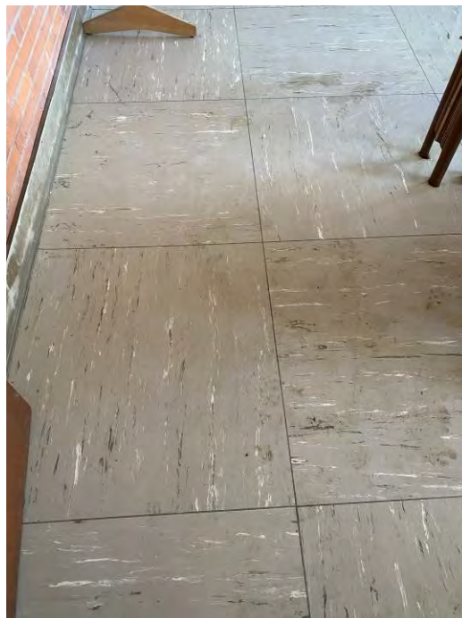
HA 12 - Tan With White & Dark Grey Streaks 3'X3' Grey Welded Seam Floor Tile No Asbestos Detected
