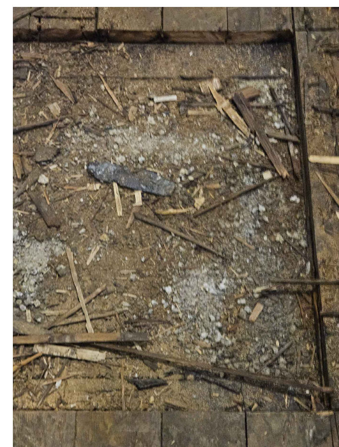
B FLY ASH WITHIN FLOORING AS VIEWED FROM ABOVE
