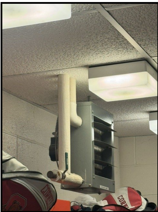
NON-ACM CEILING TILES, WHITE PAINT ON FG ENDS
