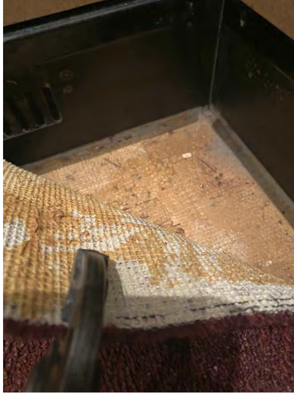
HA 13 - Elevator Cab Carpet Mastic, No Asbestos Detected
