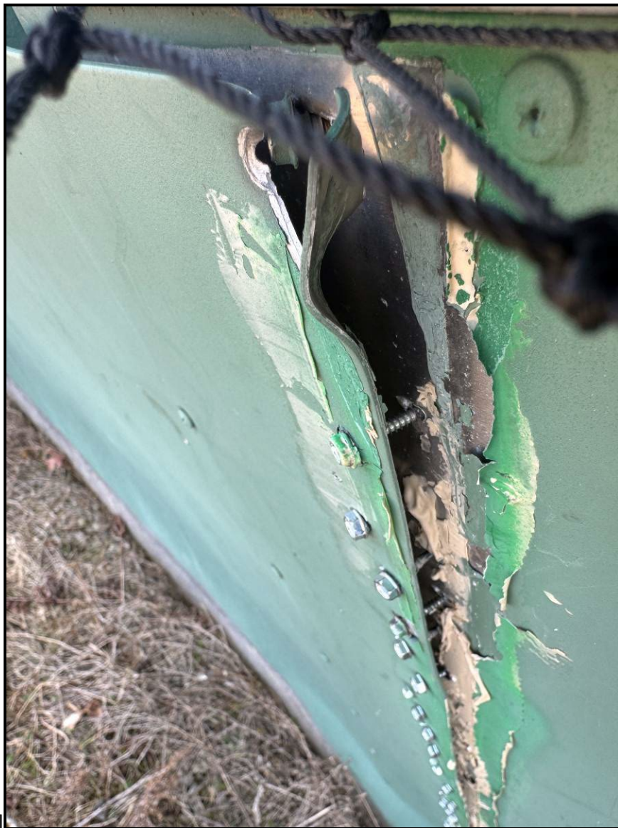
HA 01 – Exterior Metal Wall Panel Seam Caulk, No Asbestos Detected
